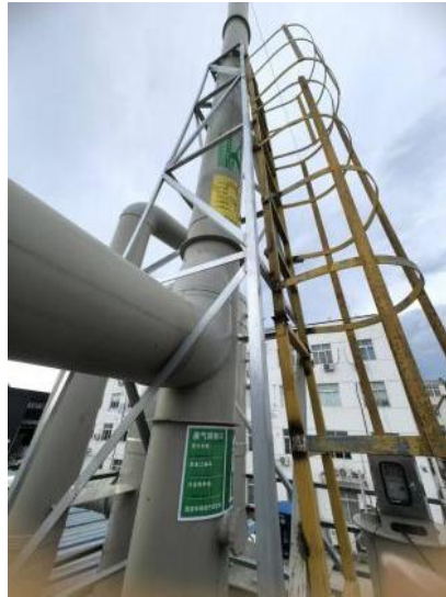
DA002 排气筒及排放口标识
